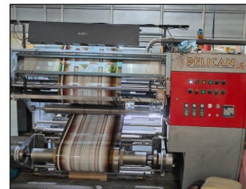
PRINTING INSPECTION MACHINE (2 MACHINE PELICAN MAKE)
